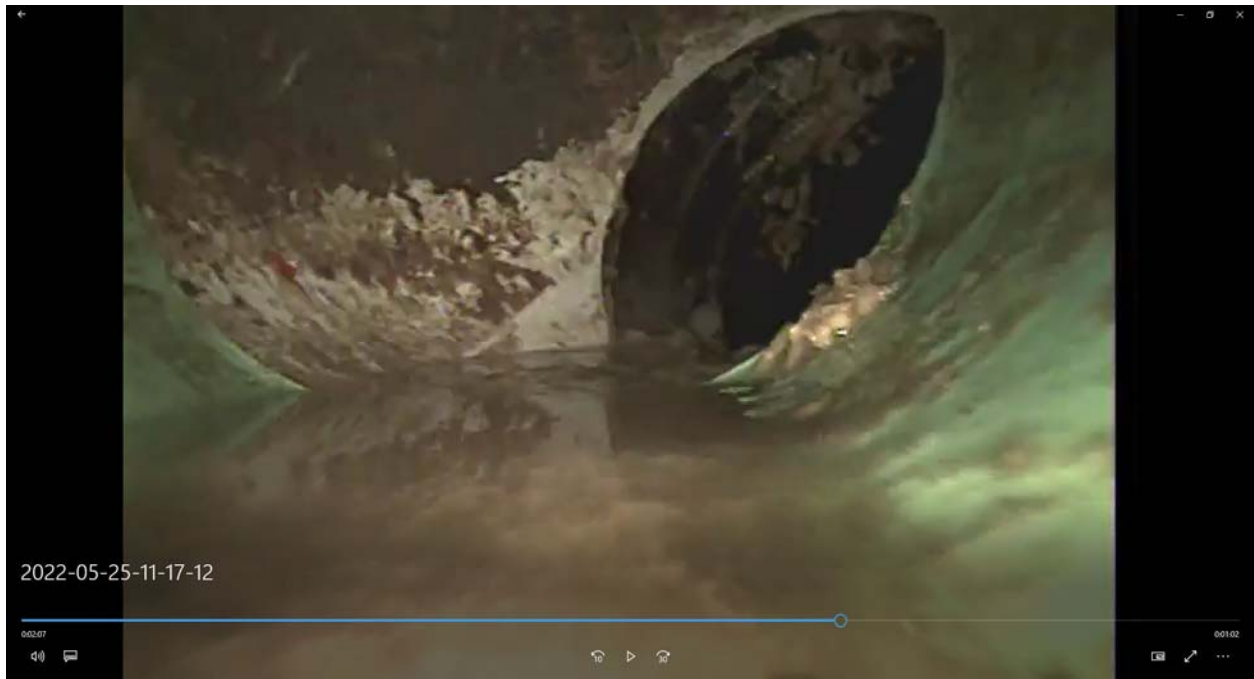
CCTV of Sanitary Sewer Lateral at 770 Shelley Parkway showing transition from PVC to VCP Pipe.
