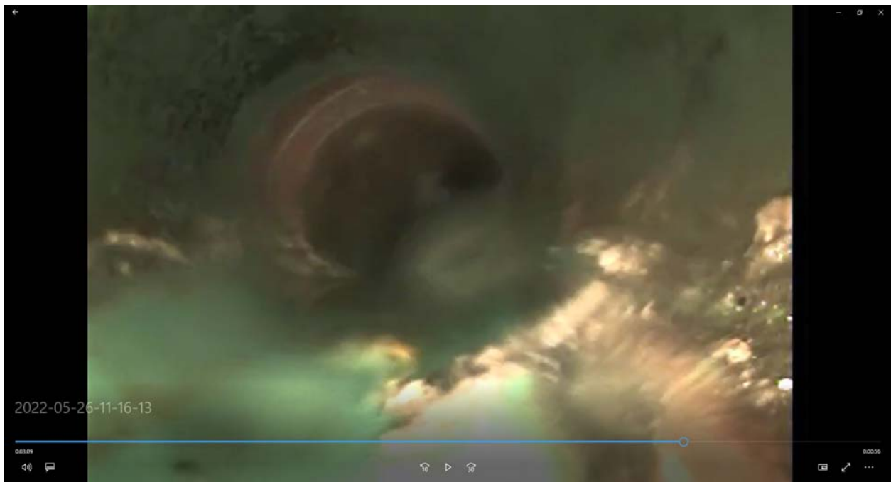
CCTV of Sanitary Sewer Lateral at 781 Shelley Parkway showing transition from PVC to VCP Pipe.
